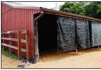
Sturdy roof gutters with downspouts direct clean water away from lot underground to grass waterway.
