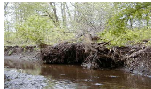
Eroded streambank at Site 17, Spring 2004
